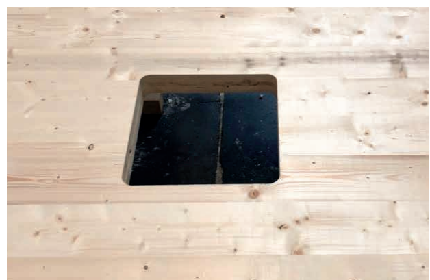
Cut-out, residual radii not removed
