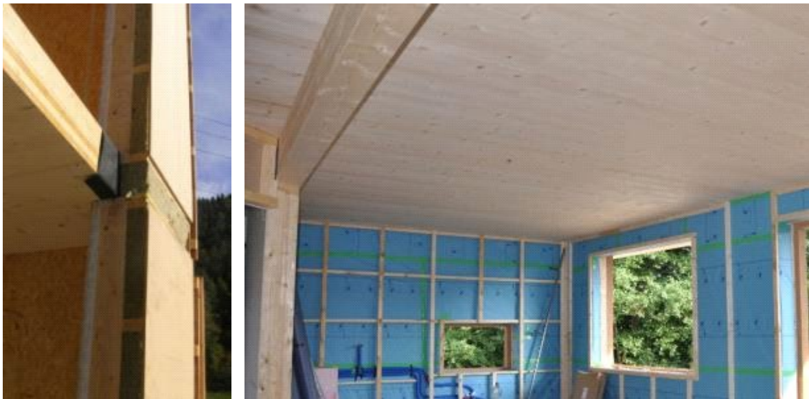
Figure 2: Combination of cross-laminated timber floor and non-load bearing external wall in timber frame constructions
