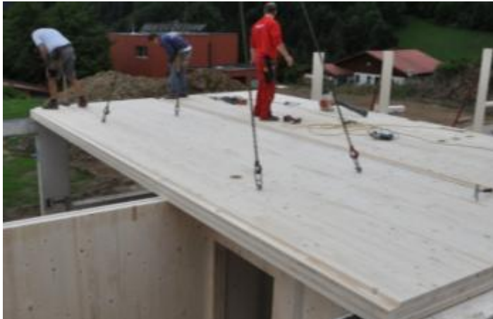
Figure 43: Continuous floors, if used with partition walls, need a suspension in order to prevent sound longitudinal conduction
