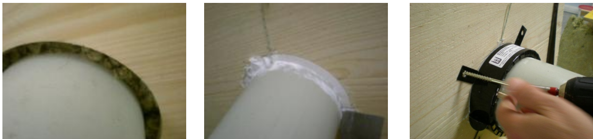
Figure 87: Installation of a fire protection collar directly in an unclad solid timber wall; left: Filling up the annular gap, center: intumescent fire protection compound, right: fastening of the fire protection collar
