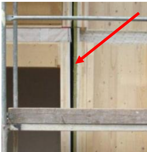
Figure 35: Stone wool and inadmissible continuous air layer between partition walls
