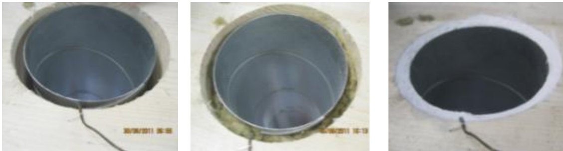
Figure 90: Insulation of the annular gap between ventilation pipe and wooden component with stone wool (center), application of an intumescent fire protection compound with a depth of about 15mm (right)
