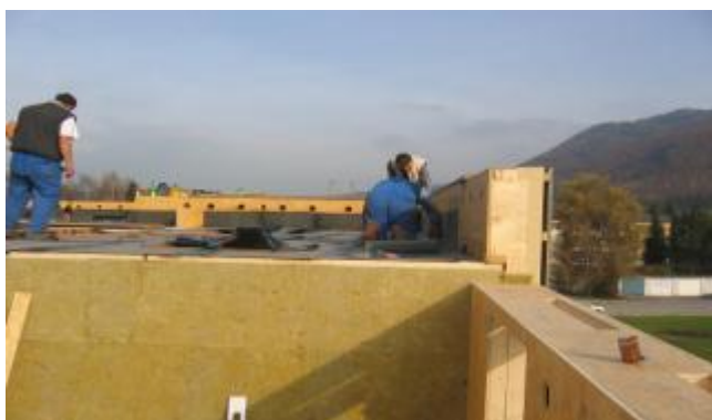
Figure 46: Vapor retarder (bituminous sealing) on a flat roof as a required weather protection
