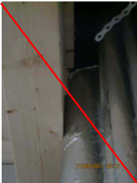
Figure 79: Incorrect execution: Due to a later extension of the shaft, non-combustible cladding of the wooden beam inside the shaft is not possible
